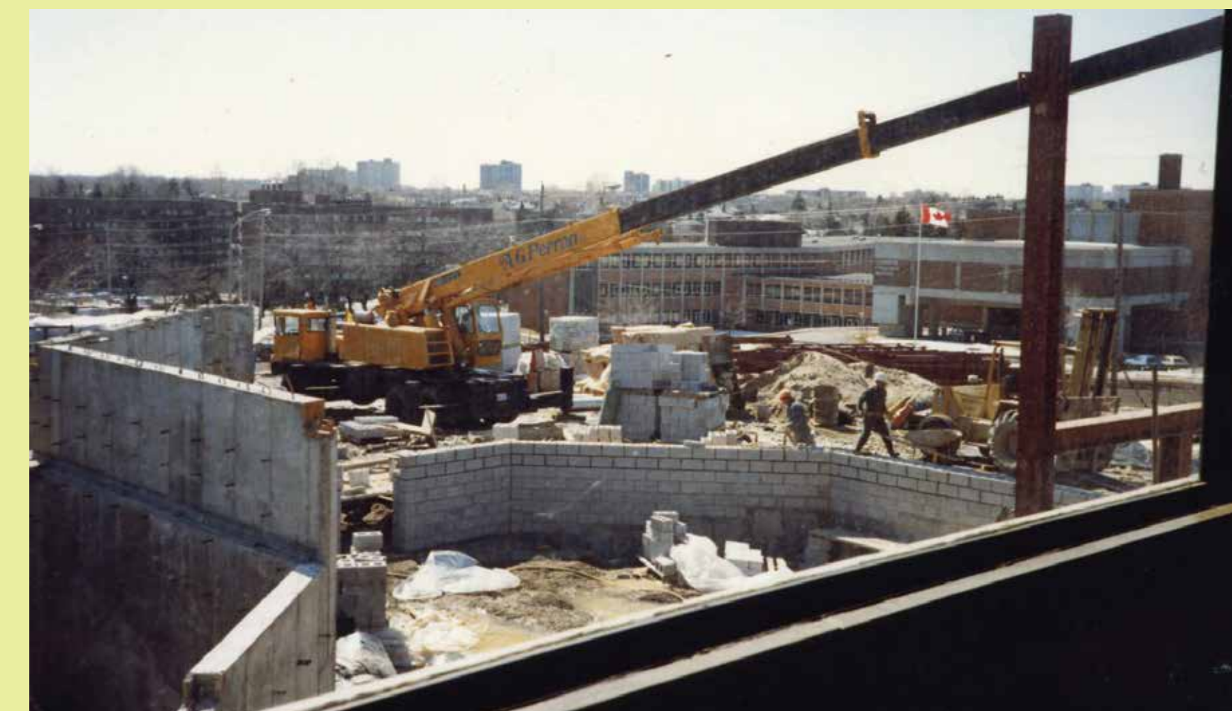
Construction of the extension, looking west, spring 1982. The extension was added to the south part of the building.
